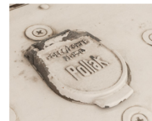
External Power Receptacle
