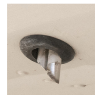
Heater Fuel Drains
